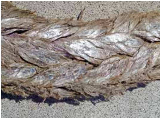
Excessive abrasion wear – volume of total rope in selected area is substantially reduced
