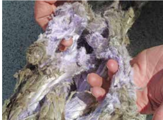
Excessive interior abrasion wear
