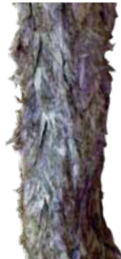
Discoloration and Burns
