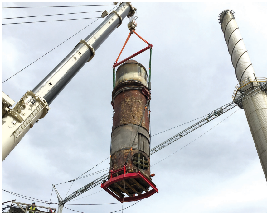
The heat exchanger during vertical lift, showing red basket frame and sling to support the aging structure.
