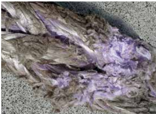
Cut adjacent strands; from its look it may have been cut by a "crossing" wire rope
