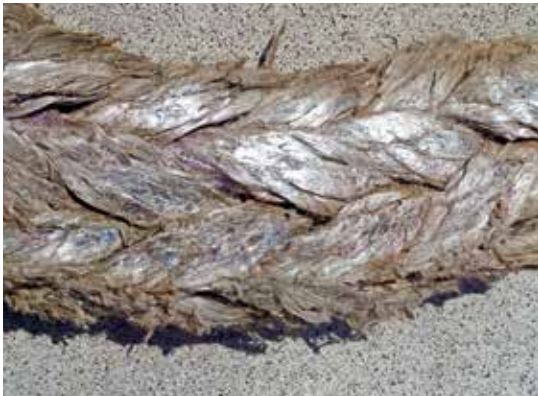
Excessive abrasion wear – volume of total rope in selected area is substantially reduced
