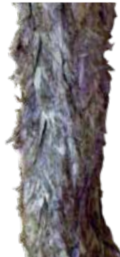
Discoloration and Burns
