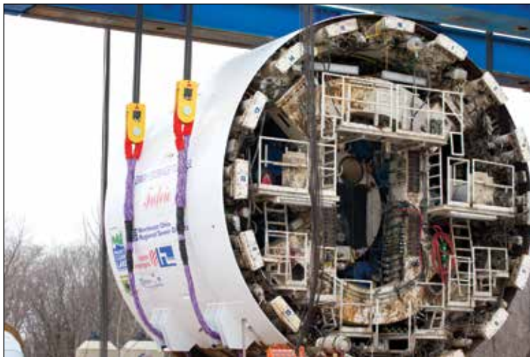
Cortland International engineered rope slings were essential in completing a major municipal infrastructure program, Project Clean Lake
